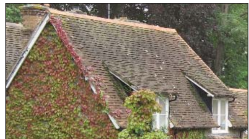
Example of where thatch has been replaced with roof tiles in Dinton
